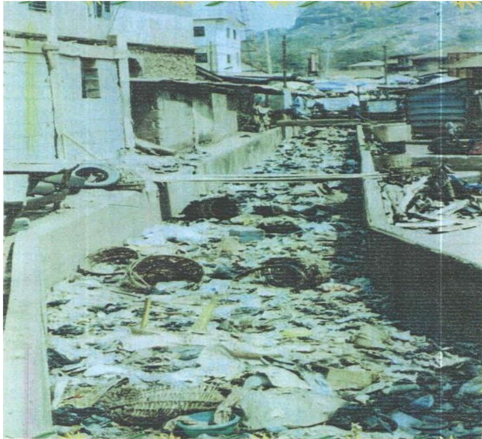
Figure 3: Refuse-clogged section of River Ajilosun channel at Odo-Otu tributary of the river. The picture was taken during the peak of dry season in February, 2018.
