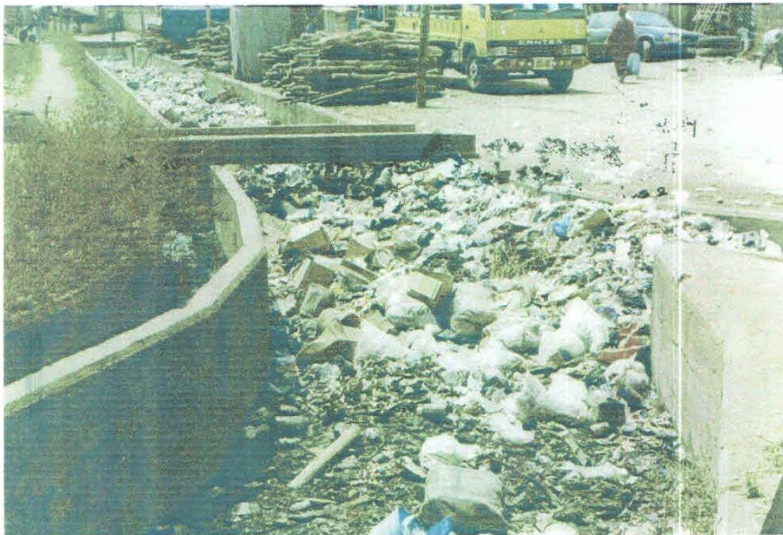
Figure 3: Refuse-blocked section of River Ajilosun channel at Atikankan in Ado Ekiti. The picture was snapped after the first few rains in March, 2018.
