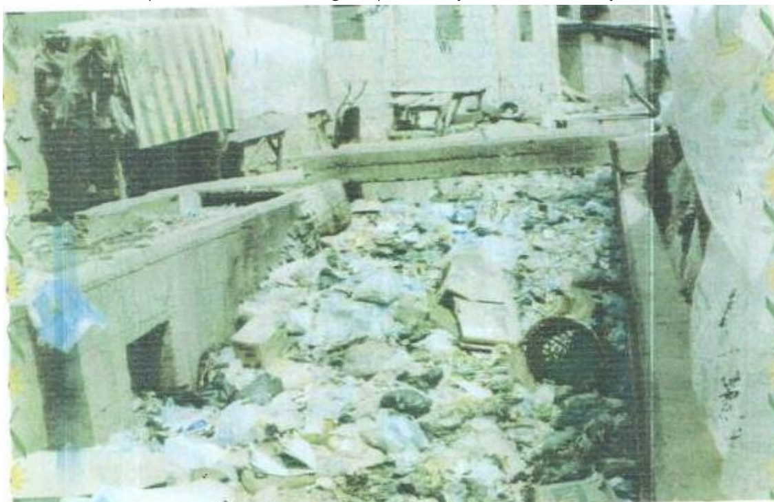
Figure 4: Refuse-choked concrete-channelized segments of River Ajilosun at Agere in Oja Oba, Ado-Ekiti.
